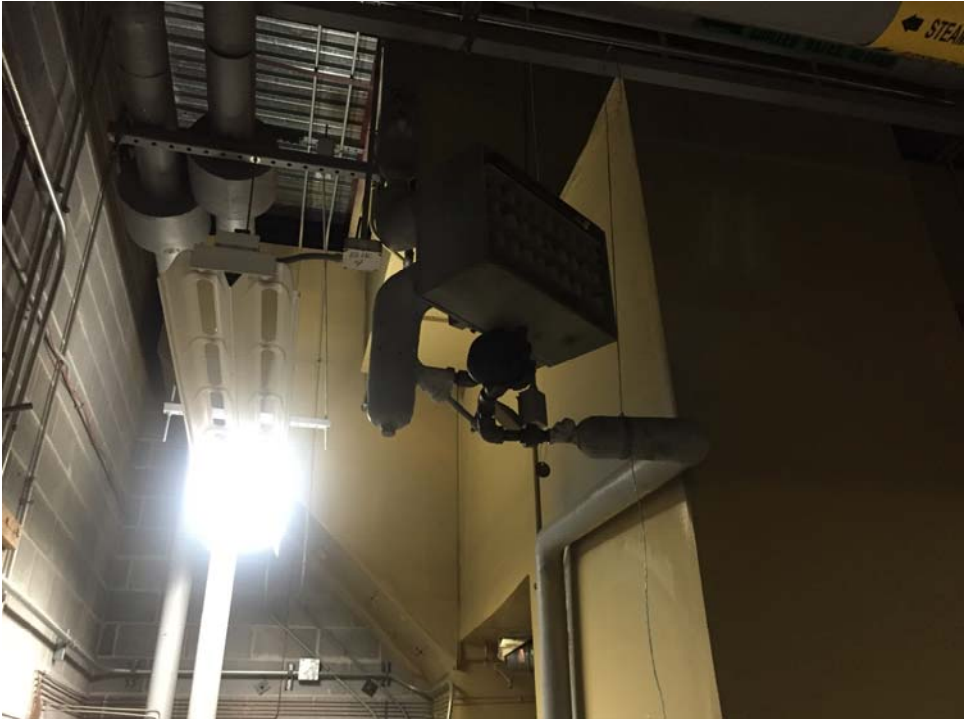
Pictures of AHU in P117:
