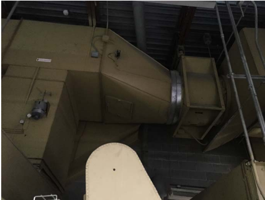
Pictures of AHU room P107:
